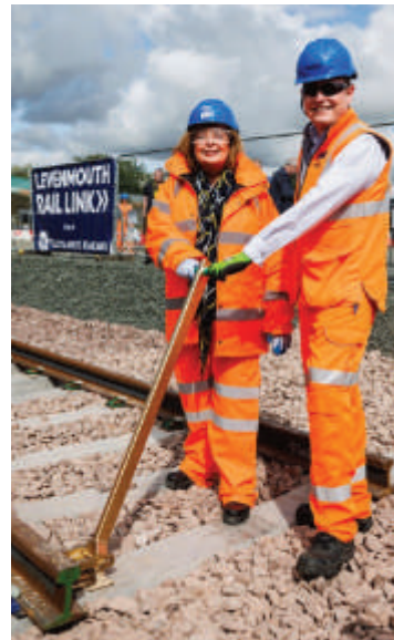
Scottish transport minister Fiona Hyslop installed the final track clip with Alex Hynes, managing director of ScotRail, to mark completion of track laying on the Levenmouth reopening project on 25 August Picture: Network Rail
