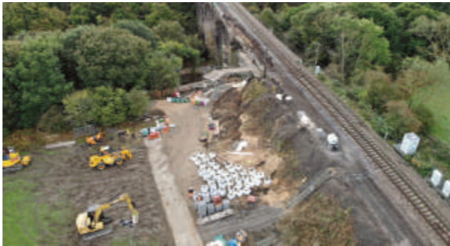
The damaged Plessey viaduct
