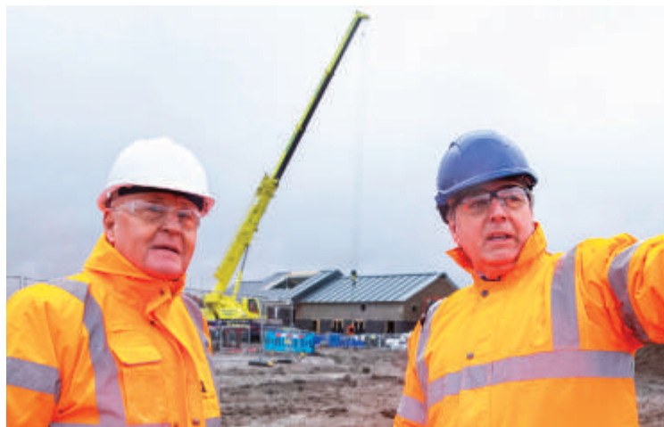
PROGRESS: Steve Rotheram (right), mayor of the Liverpool City Region, visited the site for the £80 million Headbolt Lane station at Kirkby in March with Councillor Tony Brennan. The station opens later this year and will be served by battery-electric Merseyrail trains from Wigan and Manchester
