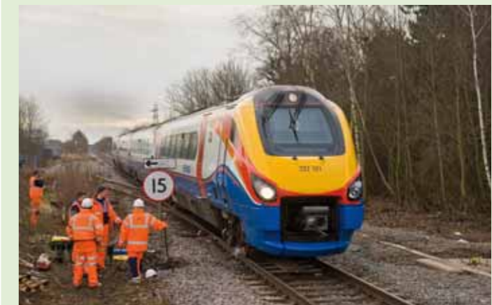
PROGRESS: Network Rail workers near Corby in January, installing five new signals which should eliminate the need for trains to retire into a siding to clear the line. One of the new signal bases can be seen on the right Picture: JIM WADE
