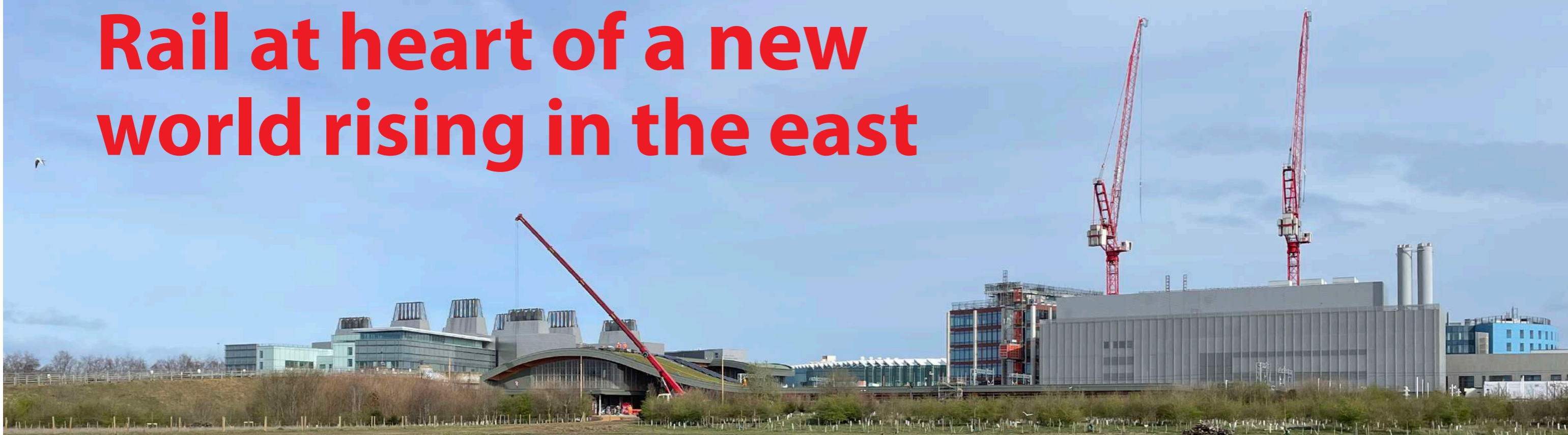
CAMBRIDGE SOUTH STATION: The curved roof of the under-construction four-track station is being given its environment-friendly sedum roof in March, just months before the official opening in June. To the right is Astra Zeneca's global headquarters and its research and development centre, one of the buildings forming the biomedical campus which employs more than 23,000 people. The campus will be home to six regional hospitals, as well as world-famous Addenbrooke's and the Royal Papworth, the Heart and Lung Institute, the Laboratory of Molecular Biology, the Cancer Research UK Cambridge Institute, the Cambridge Academy for Science and Technology, the Early Cancer Institute, the Cambridge Stem Cell Institute, the Cambridge Institute for Medical Research and the Institute of Metabolic Science
