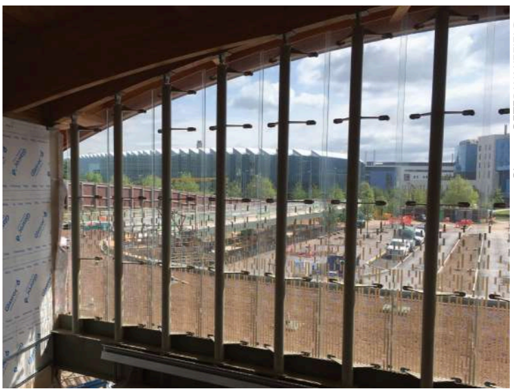
INSIDER VIEW: Cambridge South station under construction, looking out from the eastern concourse to the Cambridge biomedical campus
