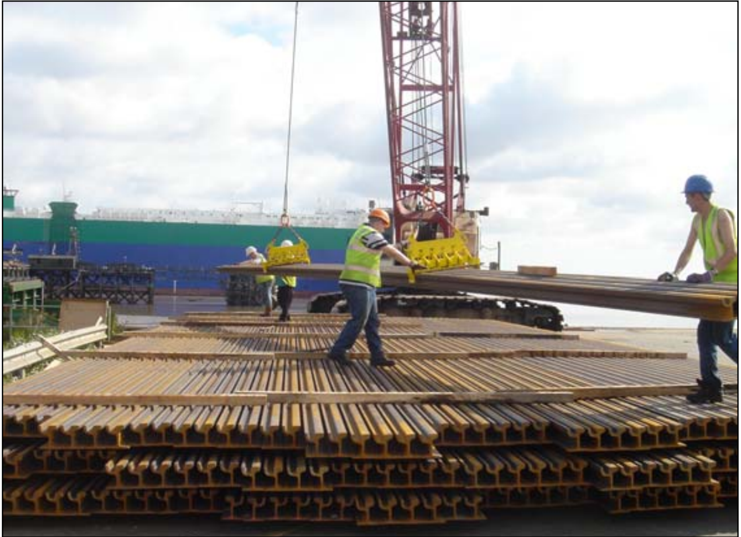
WHAT A WASTE: Rails for Merseytram unloaded at Scunthorpe before Whitehall junked three light rail projects Picture: MERSEYTRAM
